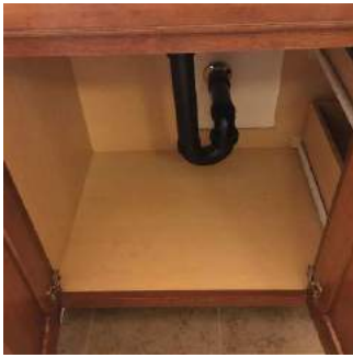
Sink & Underneath Sink (2/4) 02/02/2021 2:03 PM
