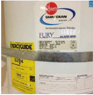
Water heater (4/5) 02/02/2021 2:12 PM
