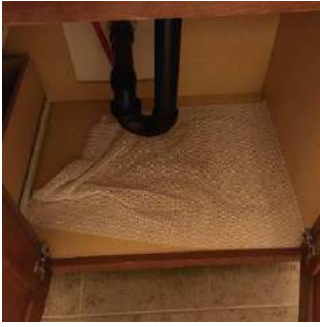
Sink & Underneath Sink (4/4) 02/02/2021 2:03 PM
