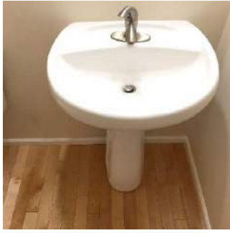
Sink & Underneath Sink 02/02/2021 1:39 PM
