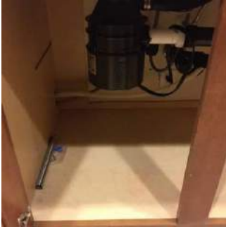
Sink & Underneath Sink (2/2) 02/02/2021 1:35 PM
