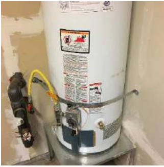
Water heater (2/5) 02/02/2021 2:12 PM
