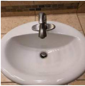
Sink & Underneath Sink (3/4) 02/02/2021 2:03 PM
