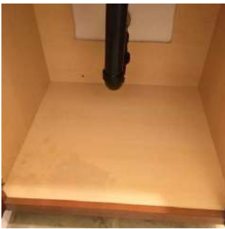
Sink & Underneath Sink (2/2) 02/02/2021 1:52 PM
