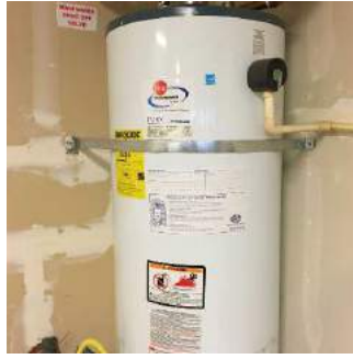
Water heater (1/5) 02/02/2021 2:12 PM
