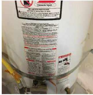
Water heater (5/5) 02/02/2021 2:12 PM
