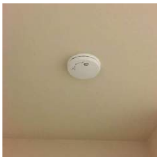
Smoke / CO detector 02/02/2021 1:55 PM
