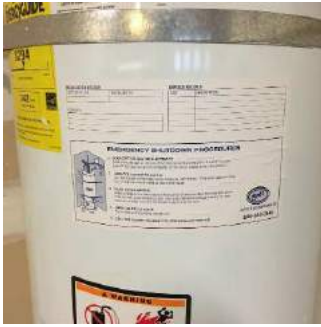
Water heater (3/5) 02/02/2021 2:12 PM
